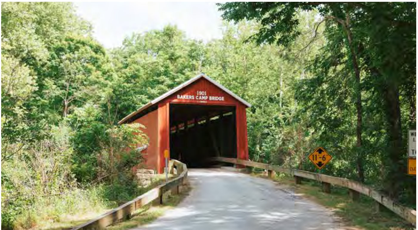
Bakers Camp covered bridge over Big Walnut Creek along E CR 650 N, east of Bainbridge.
